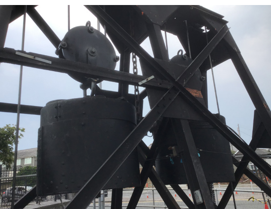
Gantry sheave in-situ
