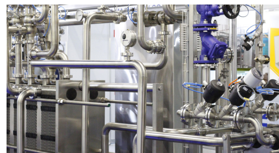
Dairy tubular heat exchanger
