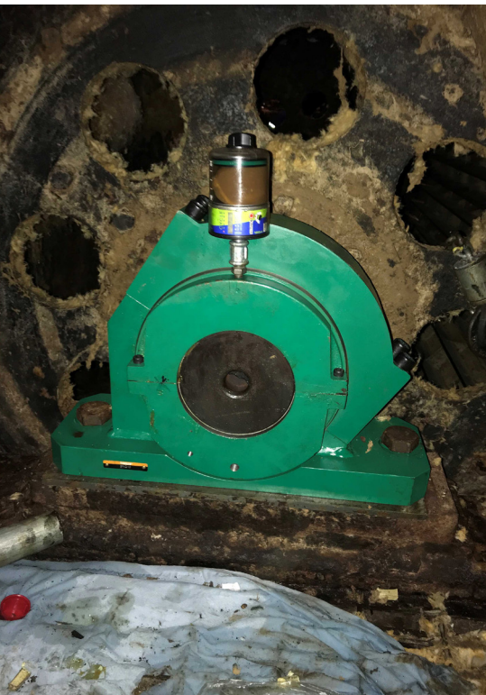
SNQ Diagonal Split Bearing in-situ
